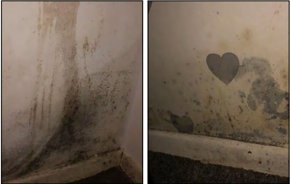
Figure 1: Mould on the wall of a child's bedroom, Langley, 2023
